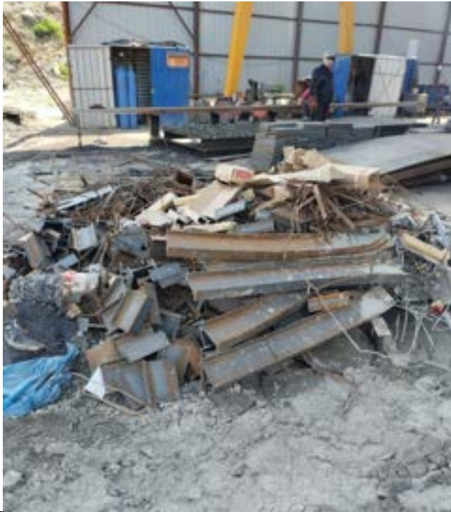
Poor Waste Management (Interchange 2, April 2023)
