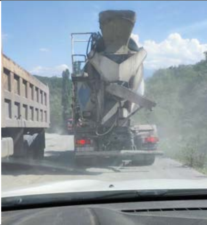
Poor Dust Management (Access Road to Tunne 4&5, June 2023)
