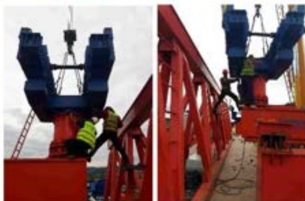
Picture 10: Non-compliances (Work at height Safety-Possible injury of working personnel) (Bridge 4 – Interchange 2) Violation of work at height safety standards has been observed by the Engineer, when inspecting the work process. The workers weren't equipped with personal safety harnesses, while platforming the task at height. The H&S and site responsible persons from the Contractor Company were informed about it. The Engineer has asked the Contractor to pay additional attention to this issue to avoid the possible incident and injury of working personnel. Non-compliance isn't solved.
