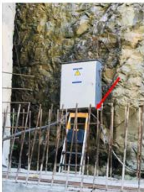
Picture 23: Non-compliance – Electrical Safety (Tunnel №5 TAA ) –Violation of workplace safety, path leading to the electrical distribution box is very unsafe, there are armatures sticking out. Safe pathway must be ensured to get to the electrical distribution box.
