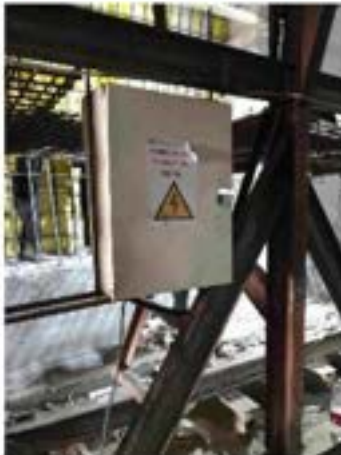
Tunnel N2AT-A – The well locked and signed up electric box has been observed.
