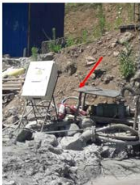
Picture 36: Non-compliance – Electrical Safety (Tunnel №4005 TA Tbilisi Portal) –Fire extinguishers are scattered around the electrical distribution box. Fire extinguishers must be placed at the proper places.
