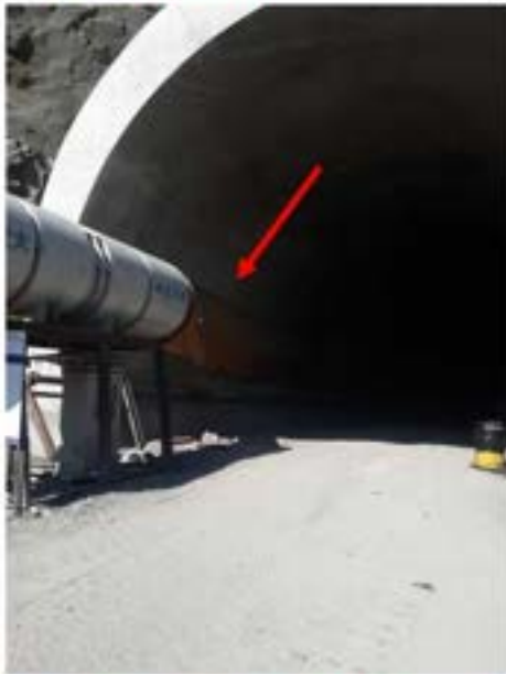
Picture 30: Non-compliance – Workplace safety Violations (Tunnel №4003 ATT ) – Ventilation is turned off and there are people working inside. It is not allowed to work in the tunnel when there is not a safe environment.
