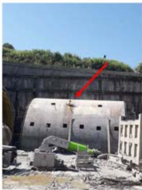
Picture 24: Non-compliance – Working at height safety Violations (Tunnel №4005 AT-TA Argveta Portal) – Violation of working at height safety requirements. Workers are not wearing safety harnesses, and personal protective equipment.
