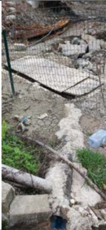
Leaking Sewage Tank (Worker's Camp No 2, March 2023)
