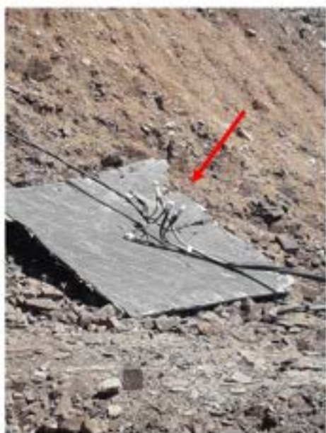
Picture 29: Non-compliance – Electrical Safety (Tunnel №4001 AT Tbilisi Portal) – Electrical wiring is not safe, cables must be checked and wiring must be safely organized.
