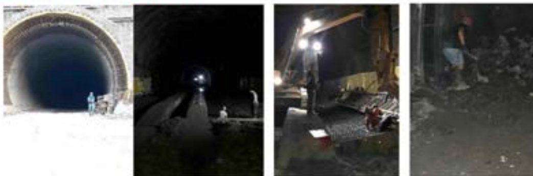
Tunnels: N4AT-A; N5AT-T; N1AT-A – Improper use of PPE by the workers when performing the task.
