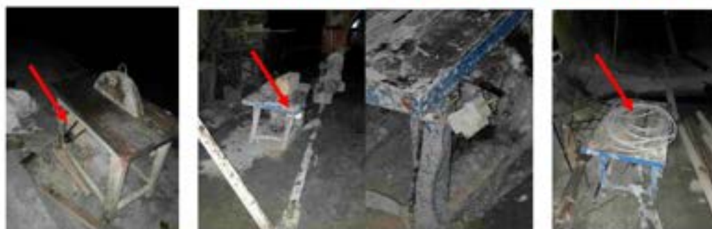
Tunnels N: 4TA-A and 5AT-T – The wood cutting machines in unsafe condition have been observed.
