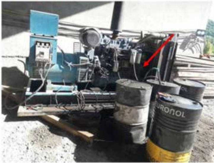
Picture 32: Non-compliance – Workplace safety Violations (Tunnel №4003 AT-T) – Generator is placed next to the fuel products, and there is no spill tray placed. Safe distance must be kept.
