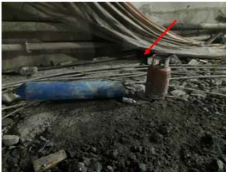
Picture 33: Non-compliance – Workplace safety Violations (Tunnel №3 AT-T) – Unsafe handling of cylinders. There is no safe distance kept between cylinders. Safe distance must be kept and special carts must be used to insert cylinders for safe handling.
