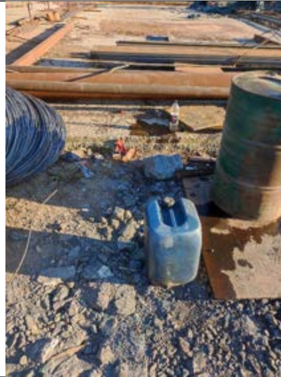
Improper Hazardous Material Storage (Steel Workshop at Interchange 2 , January 2023)
