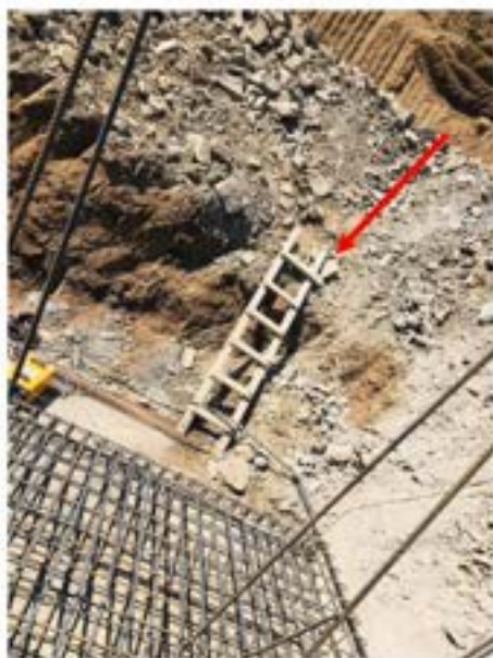
Picture 26: Non-compliance – Working at height safety Violations (Retaining wall 4501) – Homemade ladder is being used, it is not allowed to use not industrially made tools/equipment. Homemade ladder must be replaced.
