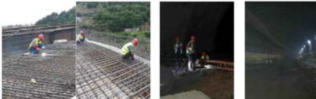
Interchange N2 (Bridge 4) and Tunnels: N3AT-A; N4AT-A: - Workers wears the proper PPE when working.
