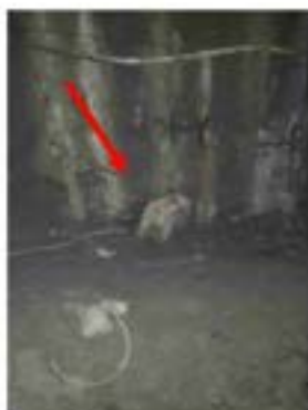
Tunnels N: 4AT-A and 4TA-A – About 1 Month this welding machine is left unattended in mud.
