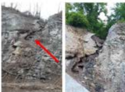
Tunnel N1AT-A – Slope is partially washed and may collapse down.
