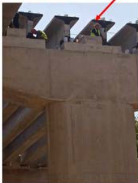
Picture 38: Non-compliance – Working at height safety Violations (Bridge №5 Pier №2 AT) – Workers are not wearing safety harnesses! Warnings regarding these violations have been given for two days and works still continued with several safety violations. These issues must be payed attention.
