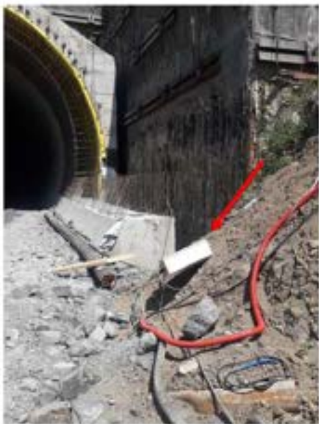
Picture 35: Non-compliance – Electrical Safety (Tunnel №4005 TA Tbilisi Portal) – Violation of electrical safety. Electrical distribution box is fallen on the ground.
