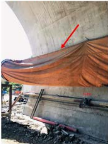
Picture 34: Non-compliance – Workplace safety Violations (Tunnel №3 ATT) – Ventilation system is turned off and there are people working inside. It is not allowed to work in the tunnel when there is not a safe environment.
