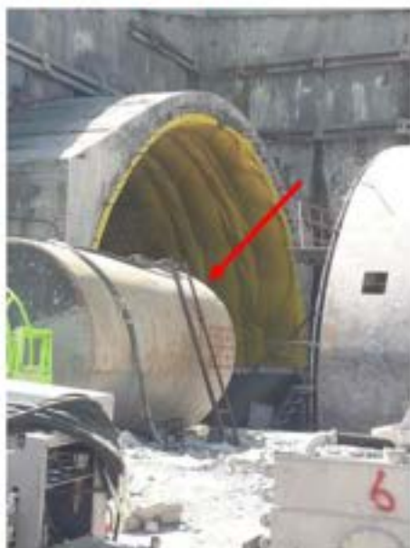
Picture 25: Non-compliance – Working at height safety Violations (Tunnel №4005 AT-TA Argveta Portal) – Violation of working at height safety requirements. Using homemade ladder, it is not allowed to use not industrially made tools and equipment.
