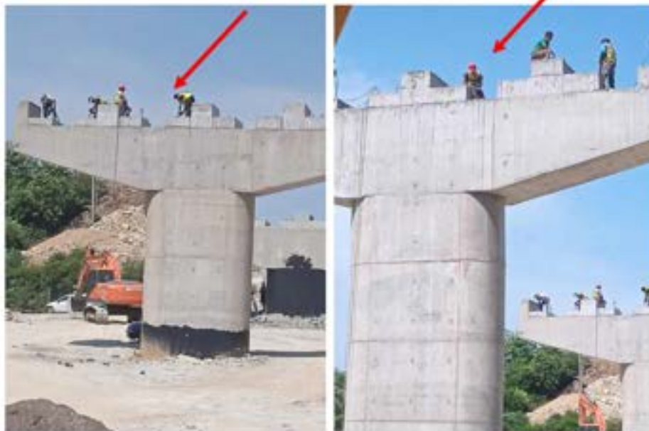
Picture 37: Non-compliance – Working at height safety Violations (Bridge №5 Pier №3 AT) –Violation of working at height safety requirements. Protective equipment is not being used when working at height, workers must wear safety harnesses.
