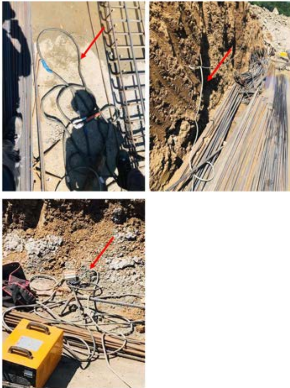
Picture 27: Non-compliance – Electrical Safety (Retaining wall 4501) –Electrical cables are scattered all around. Some of them are damaged. Damaged cables must be replaced and rest of the cables must be safely organized.
