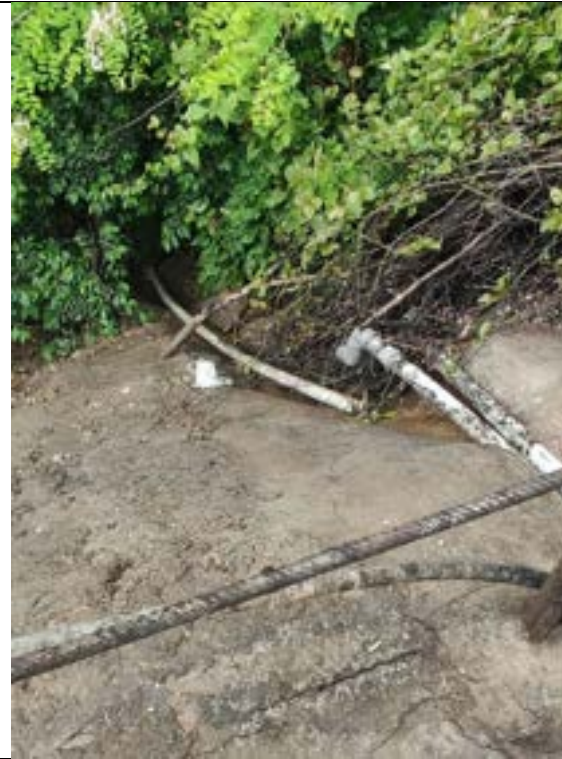
Broken Grey Water Pipes (Worker's Camp No 1, May 2023)
