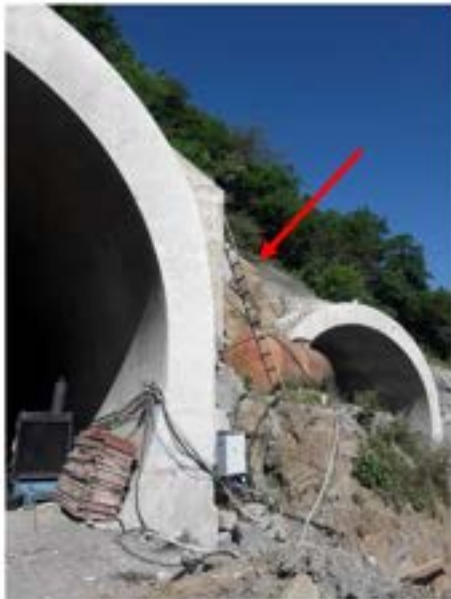
Picture 31: Non-compliance – Working at height safety Violations (Tunnel №4003 AT-T ) –Homemade ladder is being used, it is not allowed to use not industrially made tools/equipment. Homemade ladder must be replaced.
