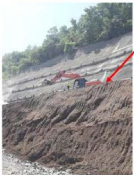
Picture 28: Non-compliance – Working at height safety Violations (Tunnel №4001 AT Tbilisi Portal) – Violation of working at height safety requirements. There are no guardrails, protective guardrails must be installed to avoid falling of people and equipment.
