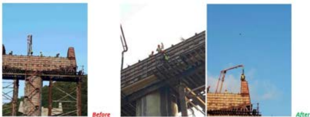
Picture 11: Non-compliances (Work at height Safety-Possible fall and injury of working personnel) (Bridge 1, Pier 2) - Violation of work at height safety standards has been observed by the Engineer, when inspecting the work process. The workers weren't equipped with personal safety harnesses, while platforming the task at height. The H&S and site responsible persons from the Contractor Company were informed about it. The Engineer has asked the Contractor to pay additional attention to this issue in order to avoid the possible incident and injury of working personnel. Non-compliance isn't solved.
