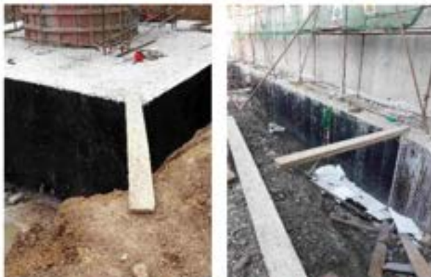
Picture 21: Non-compliance – Working at height safety Violations (Bridge N1, Pier 11 and Bridge N2 Abutment) – Unsafe accesses to the workplaces have been observed by the Engineer when inspecting the work process. The site responsible persons from the Contractor Company were informed about it. The Engineer has asked them to pay additional attention to this non-compliance in order to avoid the possible falls. Non-compliance isn't solved.
